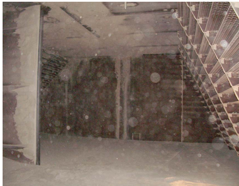
Perforated guide vanes and dividing wall for distribution to two ESP trains
