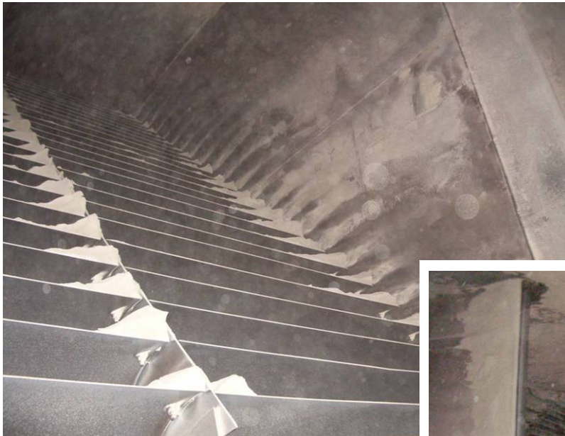
Guide vane level in duct section between air heater and ESP
