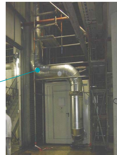
SO 3 Pipe to the injection point
