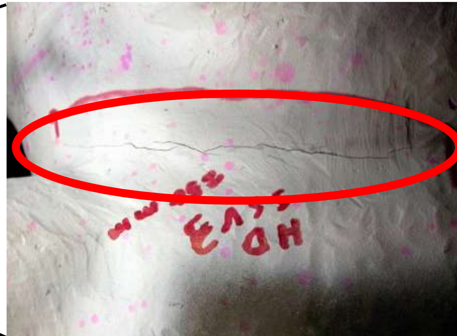
Crack depth: 50% wall thickness
