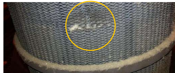
TURBINE SIDE STRAINERS DAMAGE
