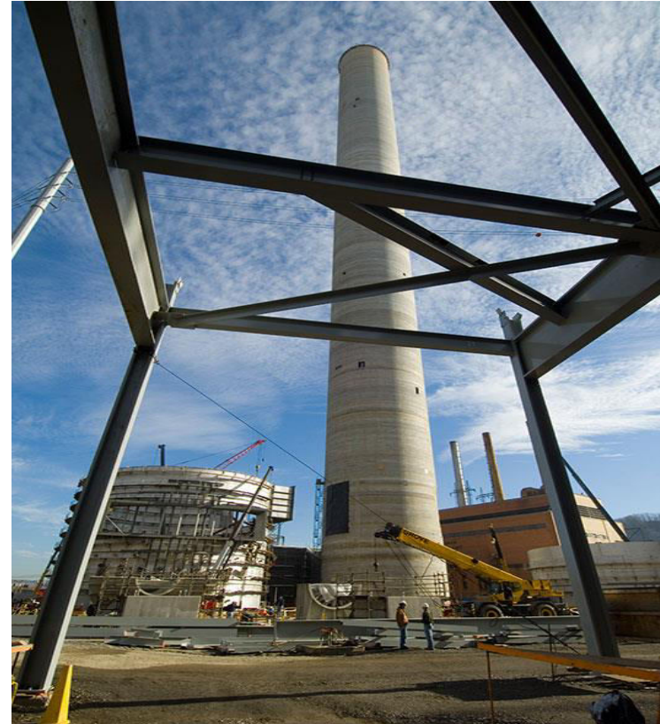
Cardinal FGD retrofit
