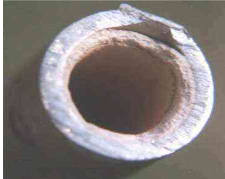
SCALING IN COOLER TUBE
