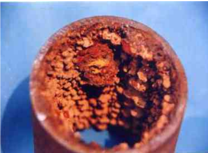
FOULING BY CORROSION PRODUCT
