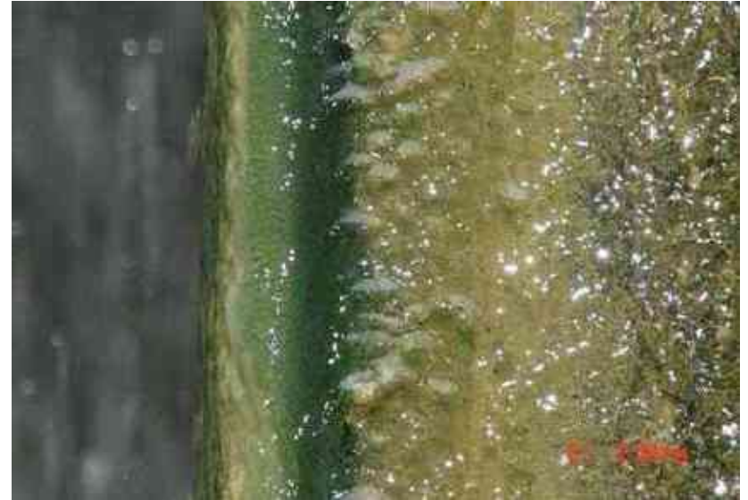
SEVERE BIOFOULING OF COOLING TOWER
