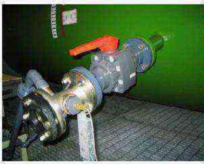
FIGURE 4 - Probe Tapping on Cooling Water Return Line
