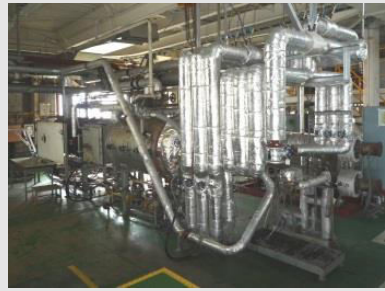
100kg/h single burner test furnace - Concept verification
