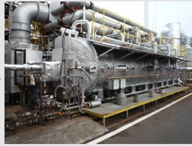
500kg/h single burner test furnace - Burner shape design
