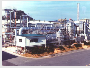
4t/h single burner test furnace - burner performance confirmation
